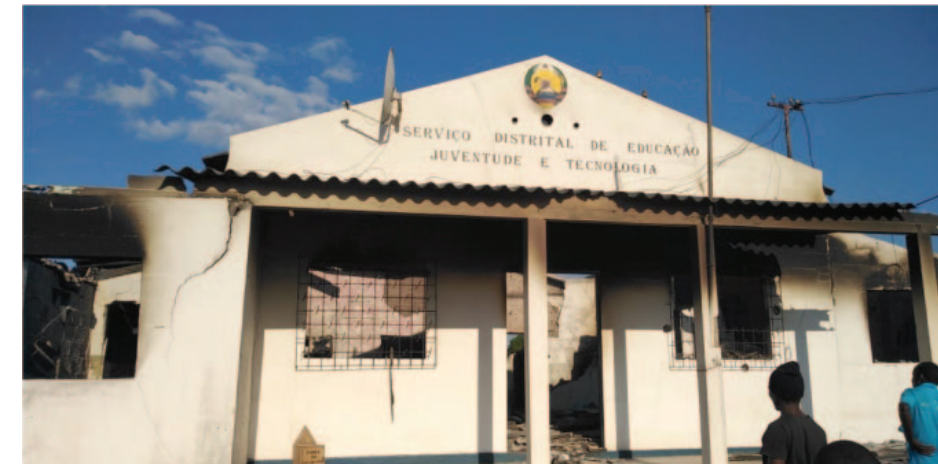
An education building in Macomia, Mozambique experienced significant damage during an attack by an armed group.
