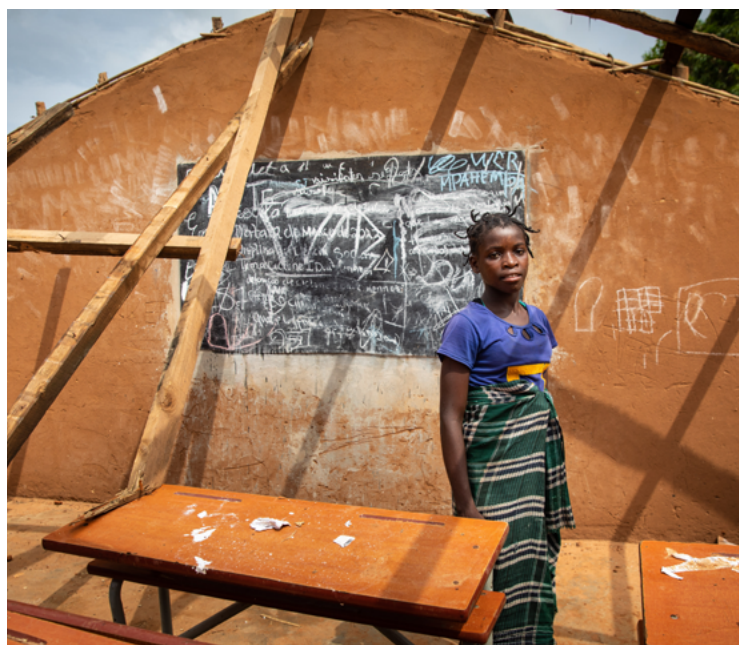
Mariano Abdala stands in front of the ruins of her school in Mozambique, destroyed by Cyclone Gombe in 2022.
